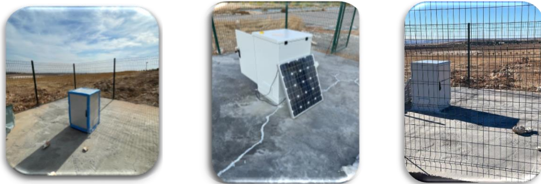
Figure 12. Supporting the Center with an Off-Grid Solar Panel System
