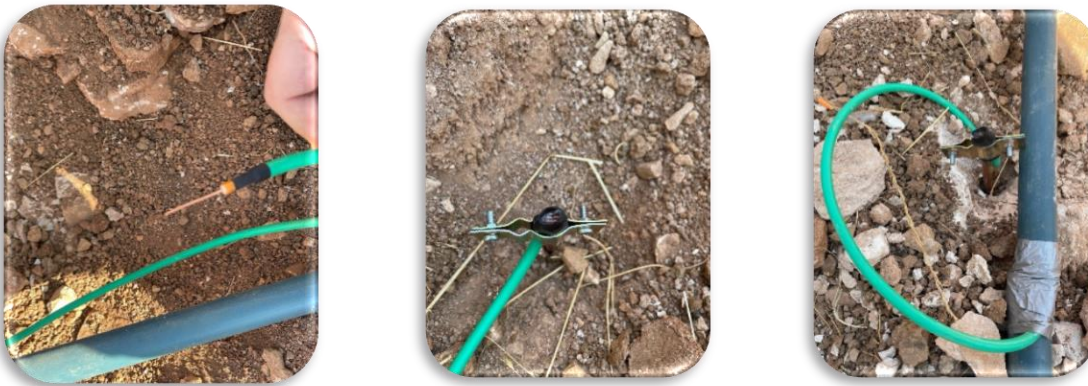
Figure 7. Connecting Coaxial Cables with Copper Electrodes
