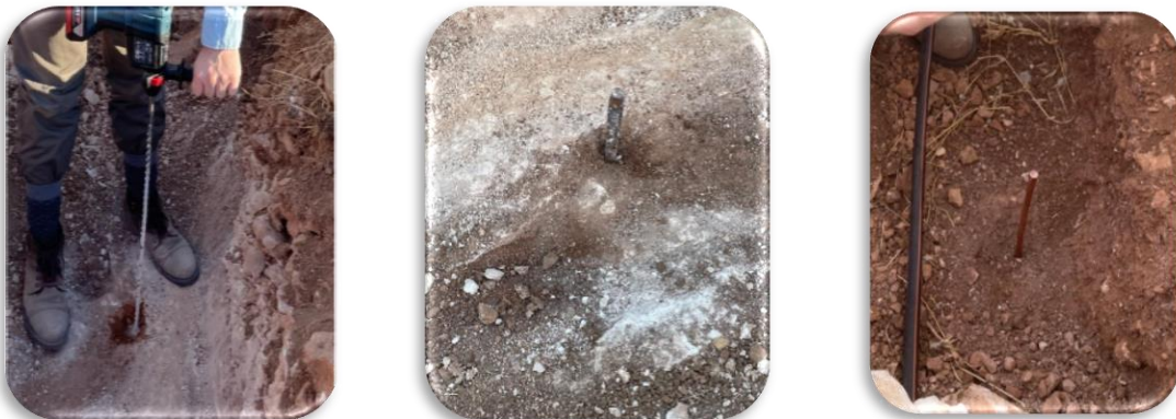
Figure 5. Copper Electrodes for Earthings
